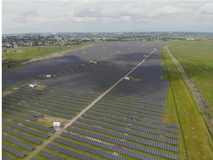
Picture 1. Melitopol solar station with power 33MW
